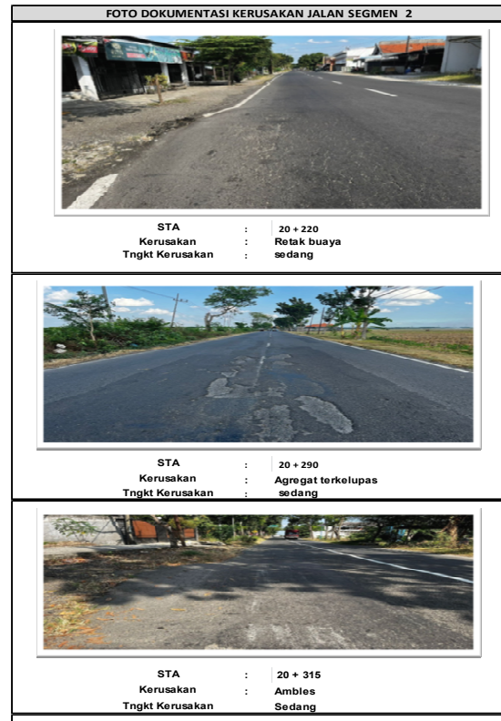
Source: Processed by Researcher, 2024 Figure 2. Segment 2 Road Damage Details
